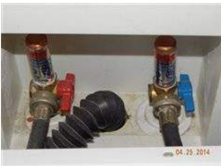
Photo 24-5 Washing machine water hookups
