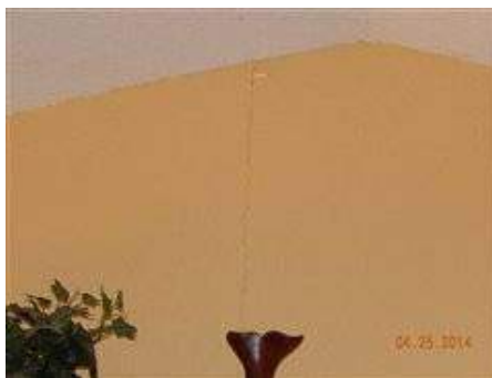
Photo 26-6 Crack in living room wall
