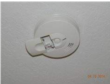
Photo 14-1 No battery in smoke detector
